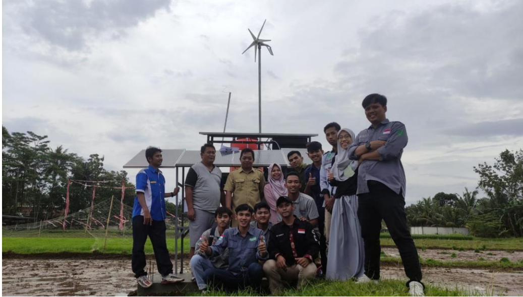
Gambar 8. Instalasi Solar Wind System Program PKM di Desa Widarapayung Wetan
